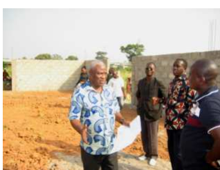
© Photo: ECOOKIM, Ivory Coast — construction of a new warehouse thanks to FT premium
